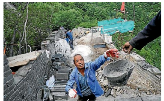
The Jiankou work is making slow progress because of the rough terrain along the 20km section being restored.
