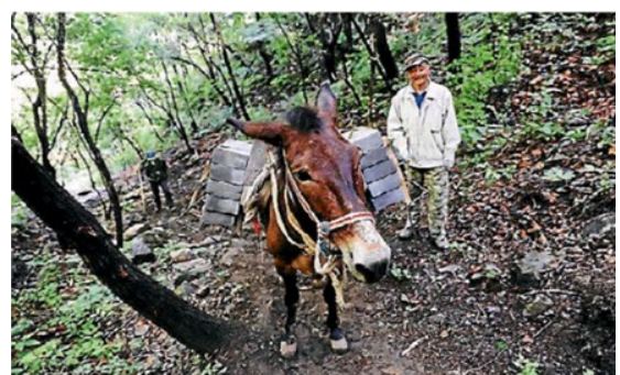
Mules have to be used to carry the bricks up the steep mountain paths to the work site.
