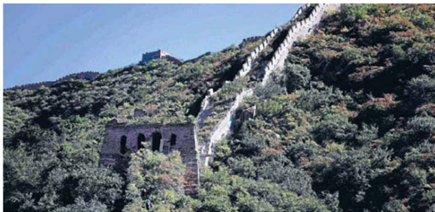
A section of the Great Wall of China that is decaying and overgrown with vegetation, located near Xiang Shui Hu village, 80km northwest of Beijing. Photo: REUTERS
